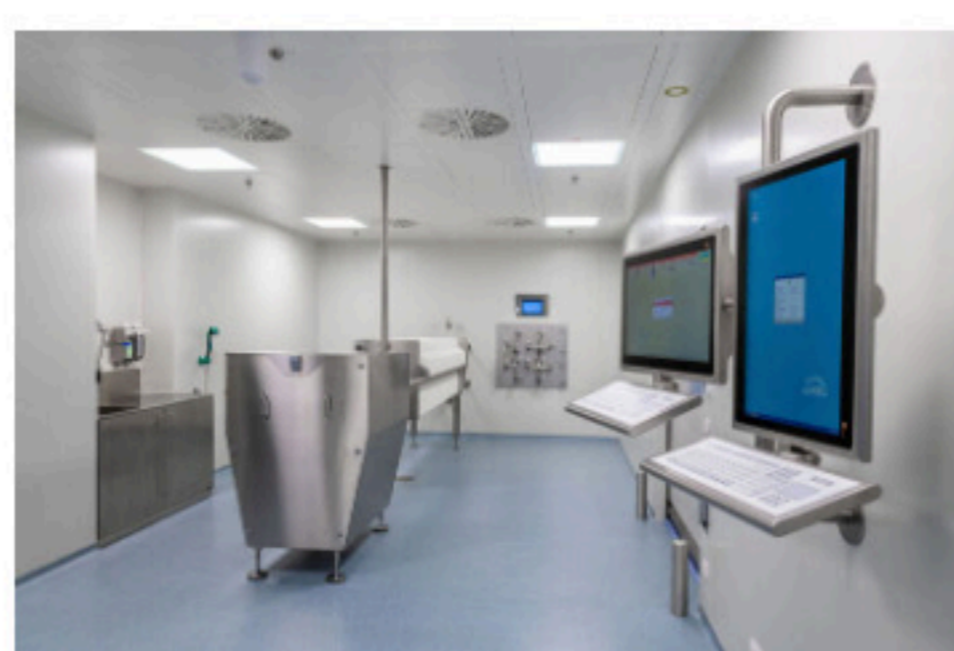
Fig. 1: Various equipment and systems installed in a cleanroom. (Source: Glatt)
