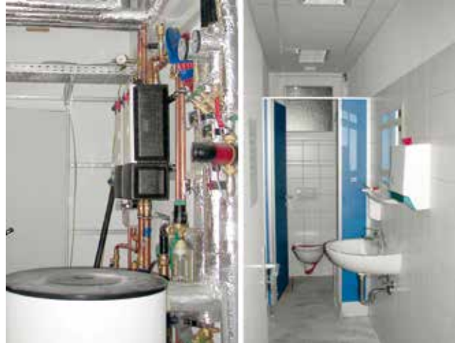
Technical and sanitary rooms
