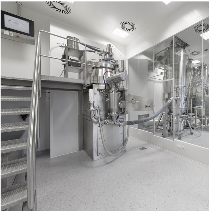
Glatt pharmaceutical plant in cleanroom design (Copyright: Andreas Suetterlin)
